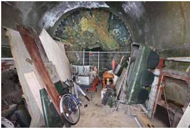
Our way forward was stopped by a fence after 16 metres. The smaller dimension unlined tunnel is soon blocked by a roof fall
